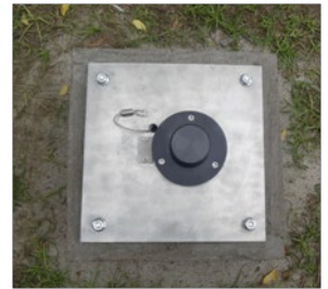
Figure 8-30: Datalogger top view
